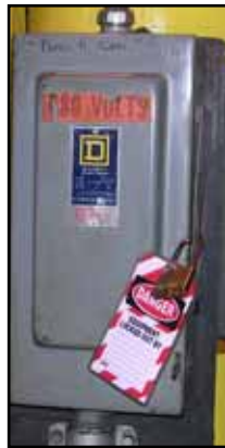
Figure 1: Lockout/Tagout on the Power Source Panel
